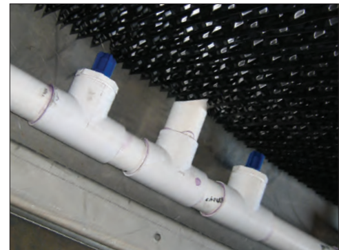
Basin Sweeper Piping
