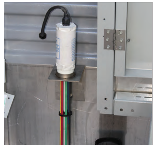
Electric Water Level Control
